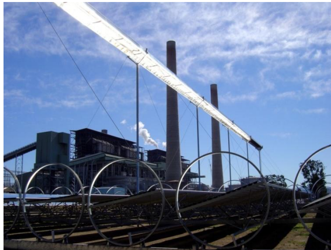
Figure 3-8: Liddell CST Collectors (picture CS Energy and Areva solar)
