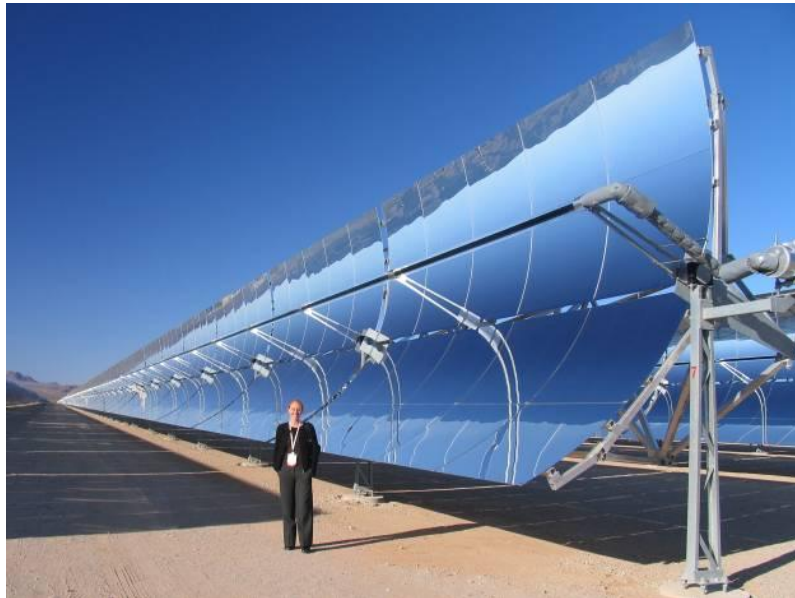
Figure 2-1: Parabolic Trough Collector (Nevada Solar 1, picture R Dunn).
