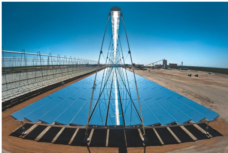
Figure 2-3: Kimberlina LFR plant, California, (picture AREVA Solar).
